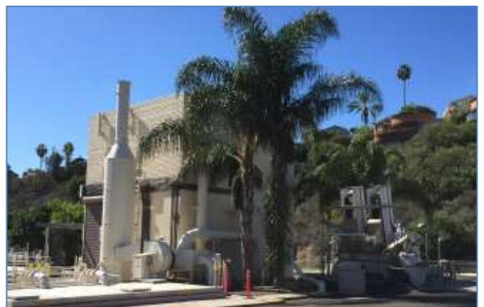
Preliminary Treatment at the SEWRF
