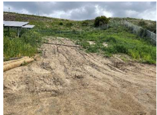
The southeast site boundaries illustrating significant erosion and rutting along the slope contributing TSS exceedances.
