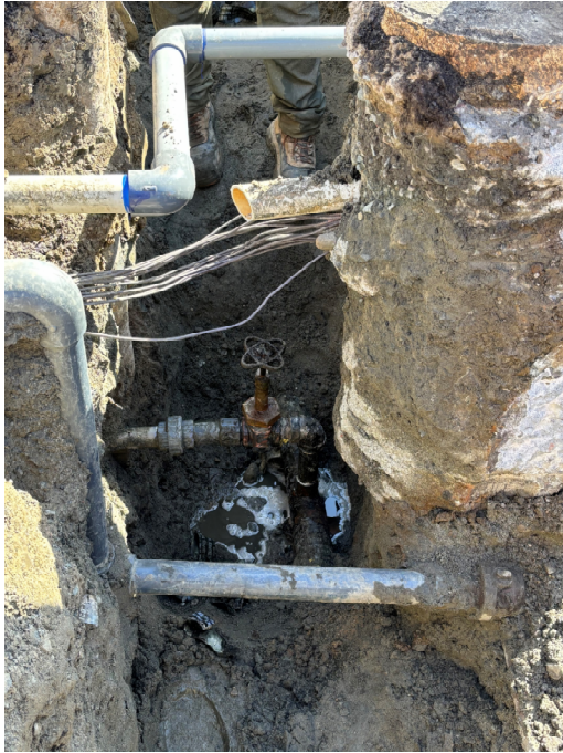
March 4, 2025 Boiler Building Lateral – location of first identified leak
