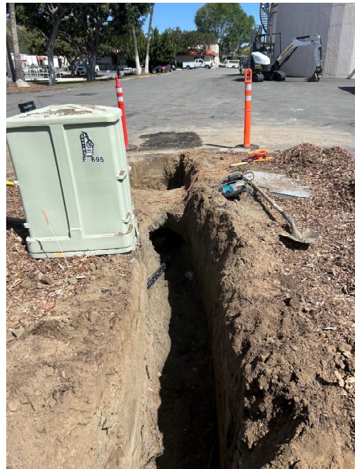
April 4, 2025 Location of damaged conduit and gas pipe below AT&T pedestal and SEJPA fiber optic handhole
