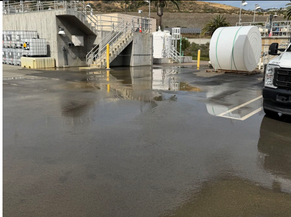
April 20, 2026 Leak Observed in Parking Lot
