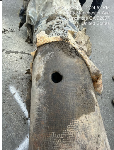
April 21, 2026 Hole in exterior of 12" ductile iron pipe
