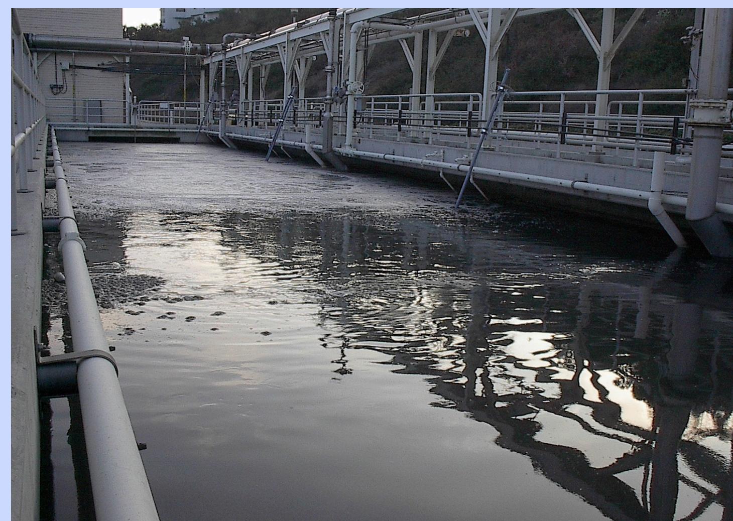
A single aeration basin (420,000 gallons) treats 3 MGD efficiently and effectively (HRT = 3.3 hours)
